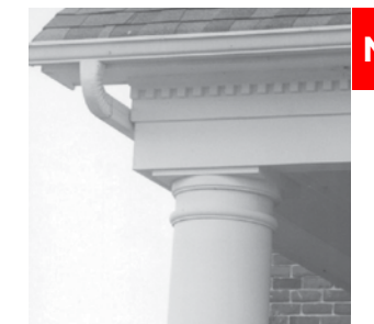
Columns which are inset or not properly aligned are always inappropriate.
