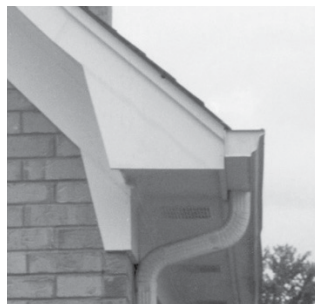
The angled fascia of this rake and frieze are not correct or appropriate.
